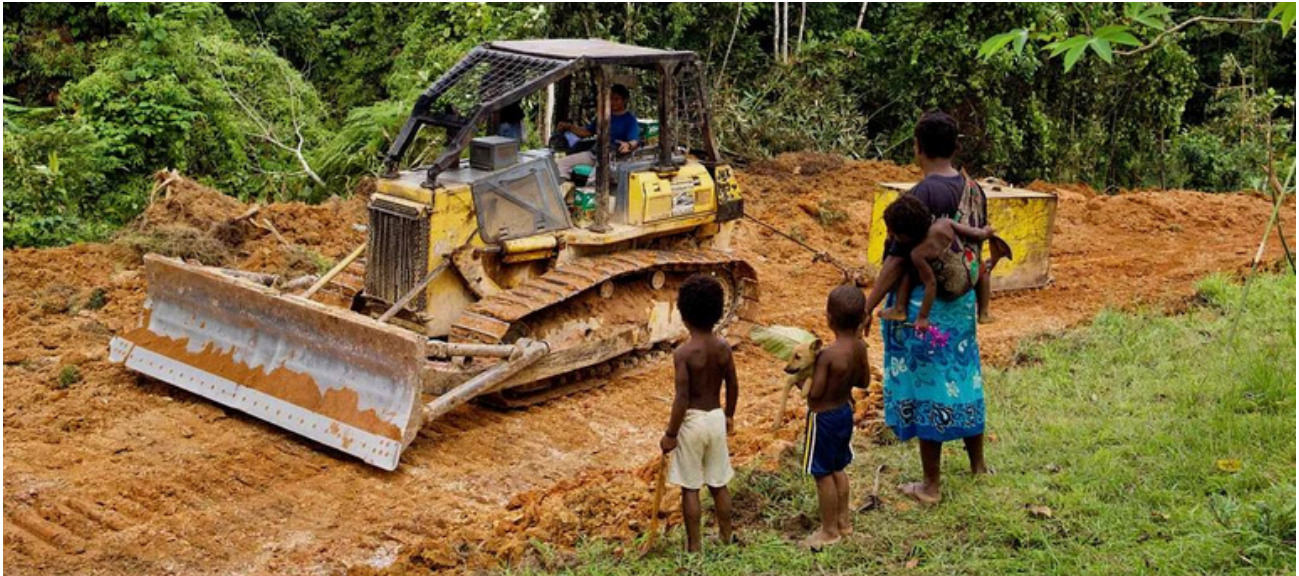
Image: Manus Island logging road under construction in Papua New Guinea. Credit: Elodie Van Lierde
